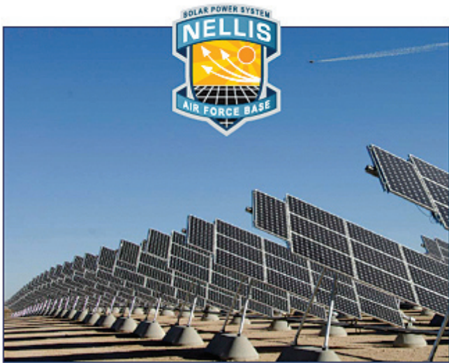
Nellis Air Force Base Solar Power System
